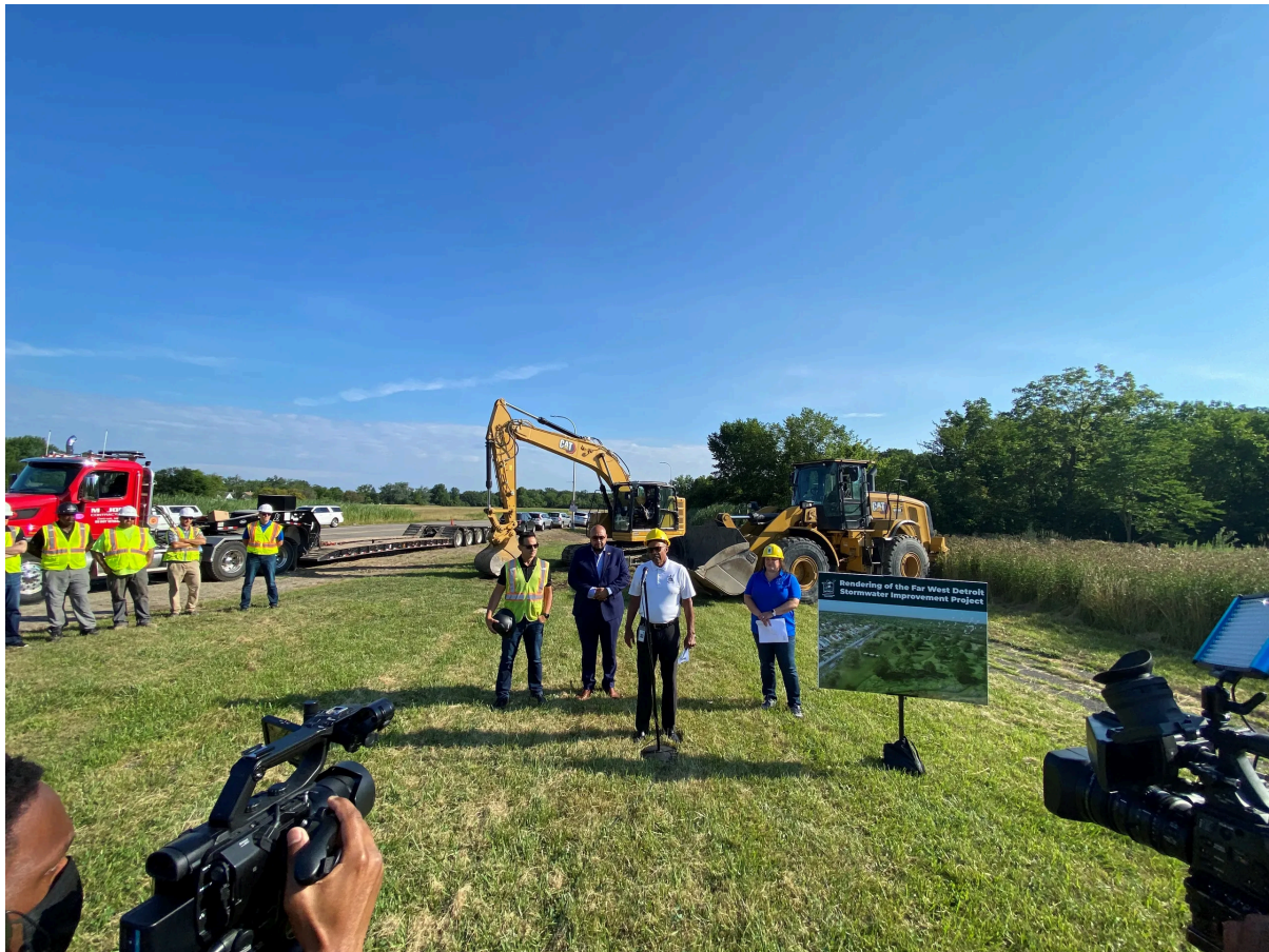
Two new detention basins will divert rainwater to prevent flooding. SARAH RAHAL, THE DETROIT NEWS
