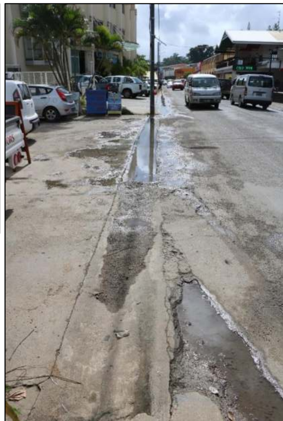
Figure 6.3 Urban drainage issues.
