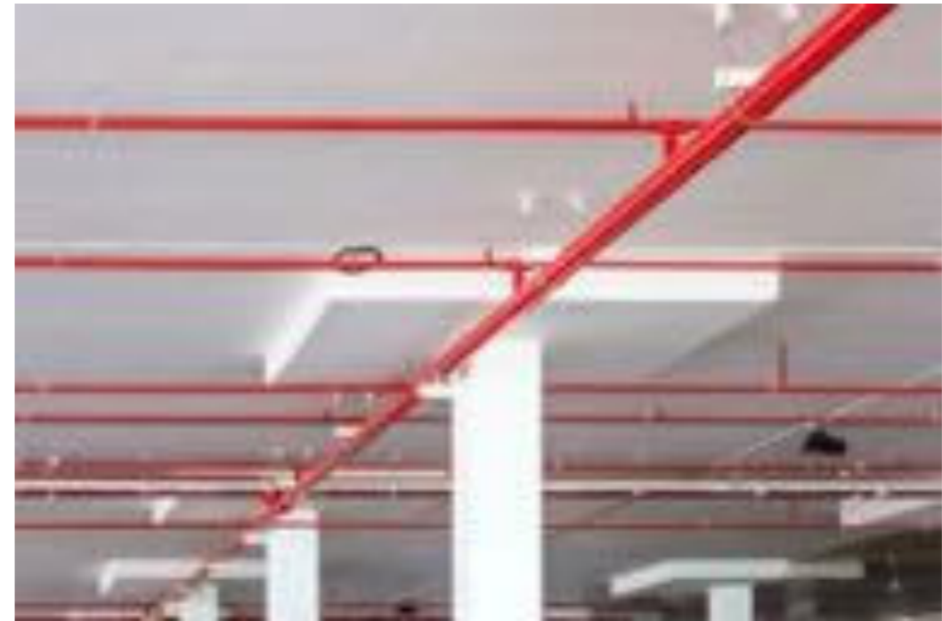
Fully Fire Sprinkler System
